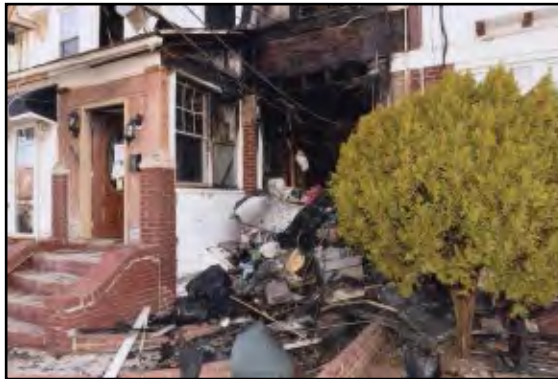
Private dwelling where arson fire occurred and which FMs James J. Egan and Andre Ramos investigated and brought to a successful conclusion.
