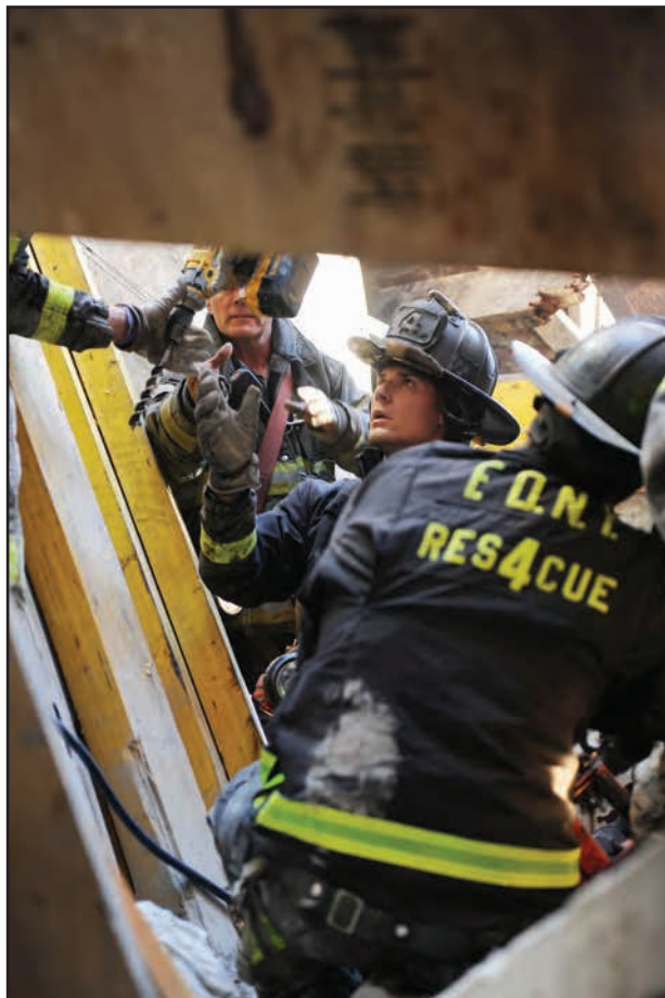
Rescue 4 members operate at collapse site.
