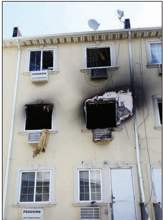
Evidence of the stubborn, two-alarm fire and the building from which Lieutenant Joseph C. Costa removed a woman and her three children.
