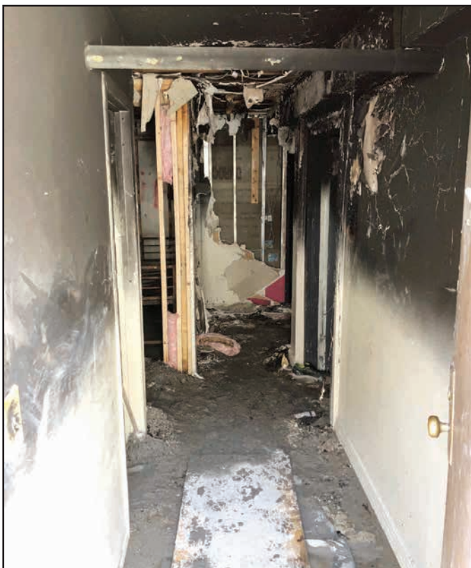
Damage to basement hallway is indicative of the conditions under which Lieutenant Hugh Barr operated.
