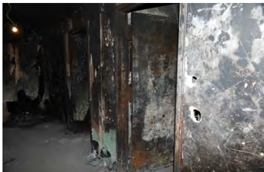
The door to the fire apartment, from the third-floor public hallway. (Photo by Bureau of Fire Investigation)
