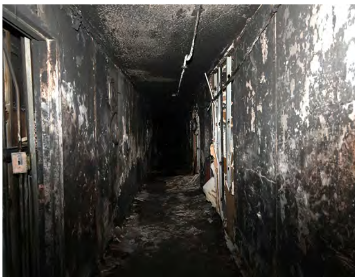
Public hallway of the third floor at Bronx Box 55-3162 on January 9, 2022. (Photo by the FDNY Bureau of Fire Investigation)
