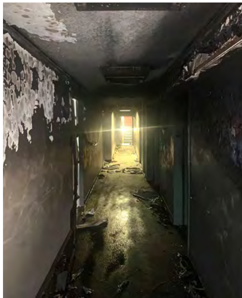
Public hallway of the 20th floor, the fire apartment floor.
