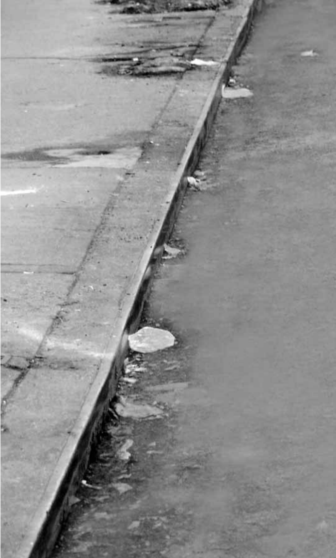
Failure to Sweep 18 Inches into the Street. See "Sidewalks and Gutters"
