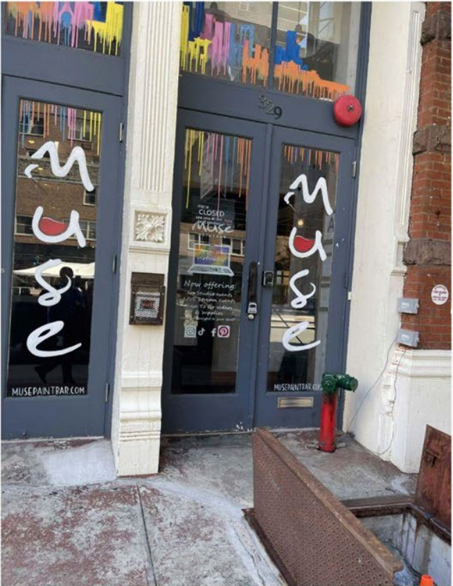
PLATFORM DAMAGE AT CELLAR HATCH DOOR
