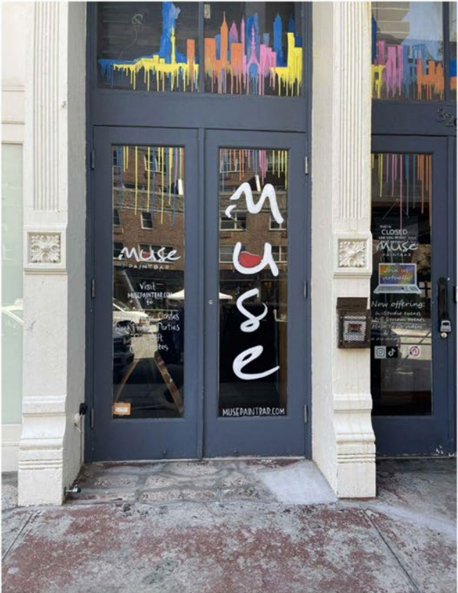
PLATFORM DAMAGE AT BUILDING ENTRANCE
