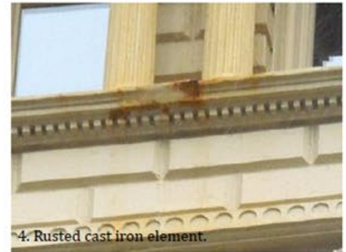
5. Damaged cast iron element.
