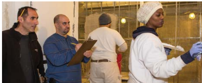
Supervising plasterers carefully watch and grade Caretaker P Contessa Evans as she applies the finish coat of plaster.
