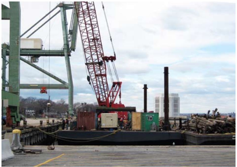
Repairing fendering and piles at Pier 9A North at the Red Hook Container Terminal.
