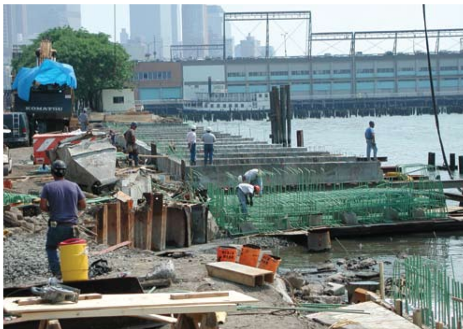
Building a public park on the shoreline, such as Hudson River Park (above), requires permits from city, state, and federal agencies.
