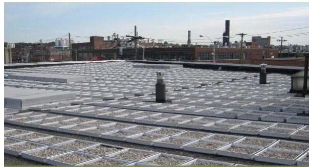
BLUE ROOF FOR STORMWATER DETENTION
