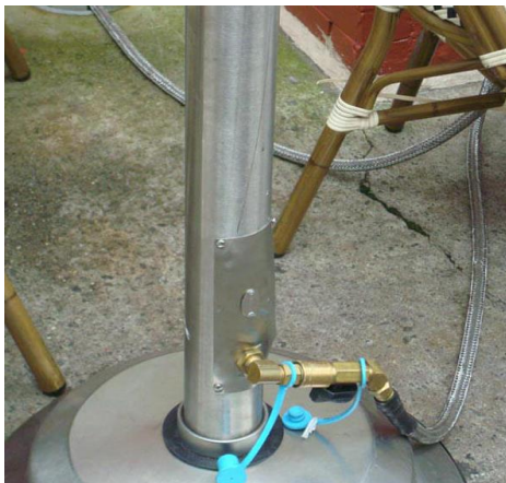
Flexible gas hose connector at portable gas heater (seen without protective cover)
