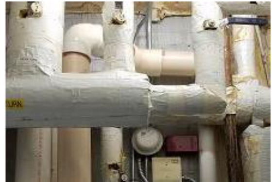
PHOTO SOURCE: Discolored unlisted PVC Vent for Category IV Boiler
