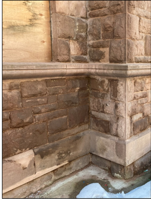
Figure 13: Water infiltration and efflorescence underneath removed window, Mulberry Street.
