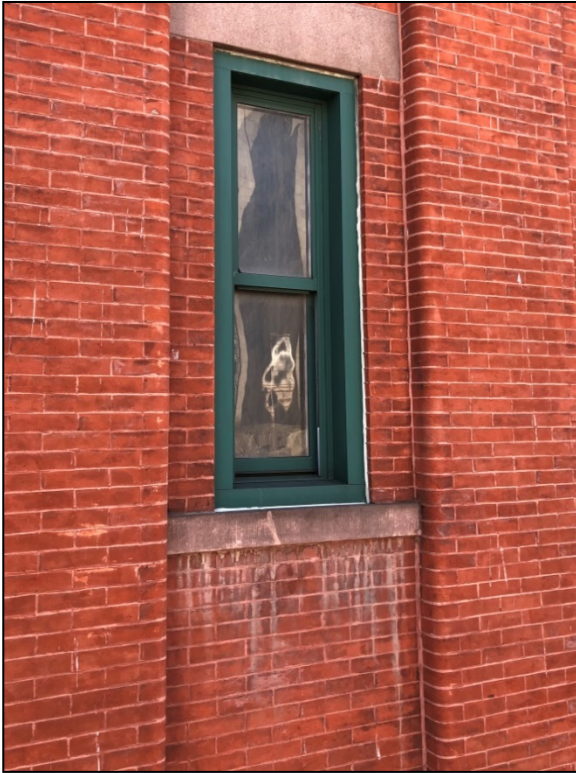
Figure 29: Atmospheric soiling and efflorescence buildup below the stone window sill stair tower, Mulberry Street.
