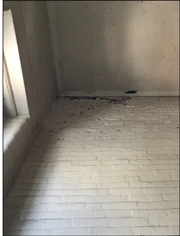
Figure 46: Fifth floor stair tower with peeling paint and efflorescence.
