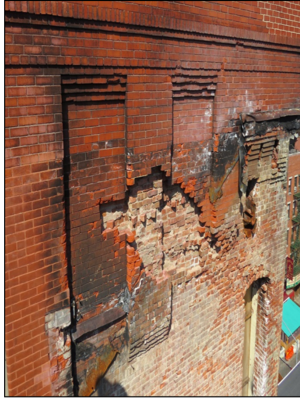
Figure 26: Fire and demolition damage, Bayard Street.
