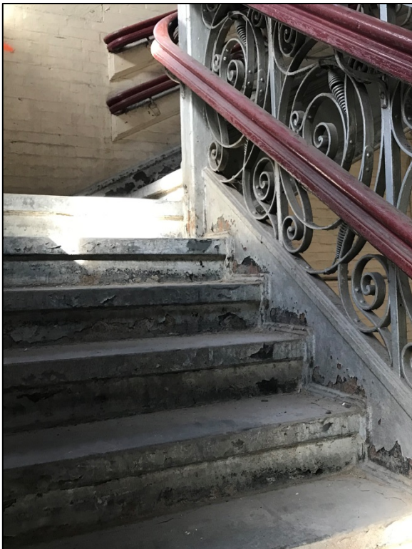
Figure 47: Stairs with peeling paint and mold.
