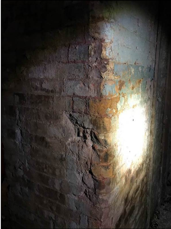
Figure 41: Pressed brick with peeling paint, mold, water infiltration, and demolition damage.
