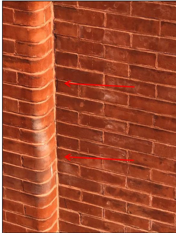
Figure 30: Crack along pilaster in masonry indicated with arrows, Bayard Street.
