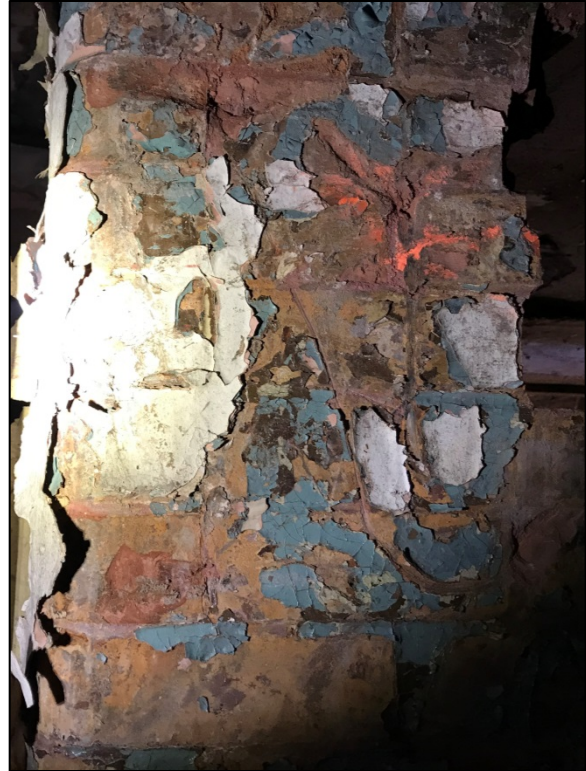
Figure 42: Pressed brick with red tinted mortar beneath peeling paint.
