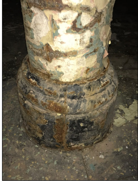
Figure 38: Corrosion at cast iron column base.
