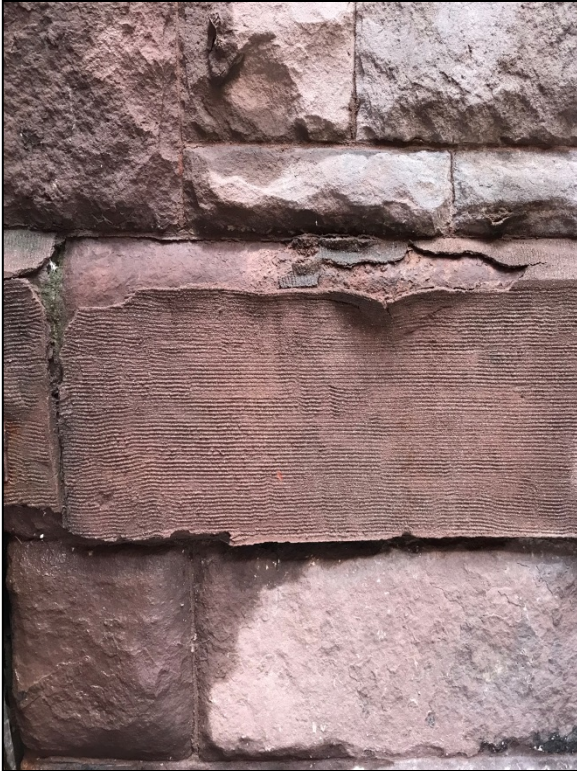
Figure 16: Delamination and water infiltration, Bayard Street.
