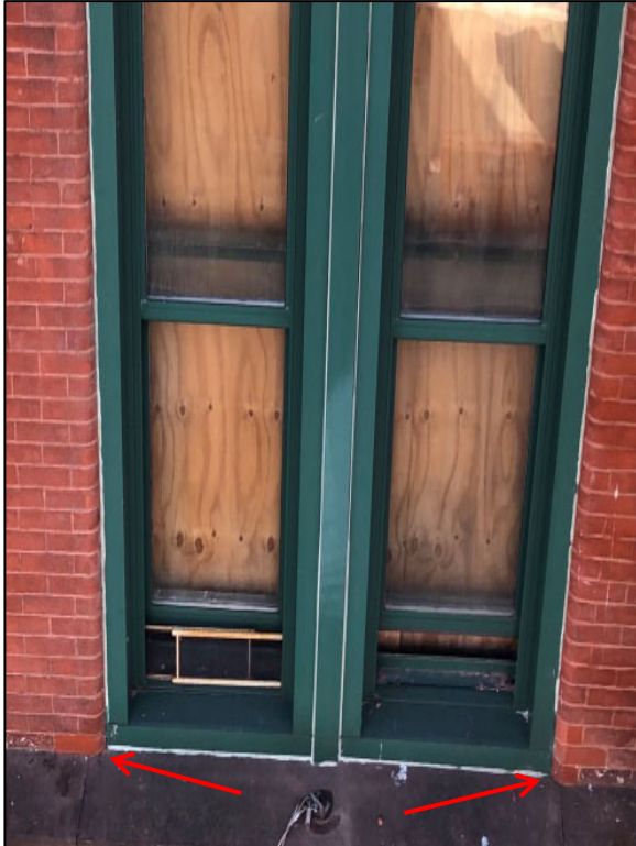
Figure 35: Replaced bricks indicated with arrows at the bottom corners of window, Mulberry Street.
