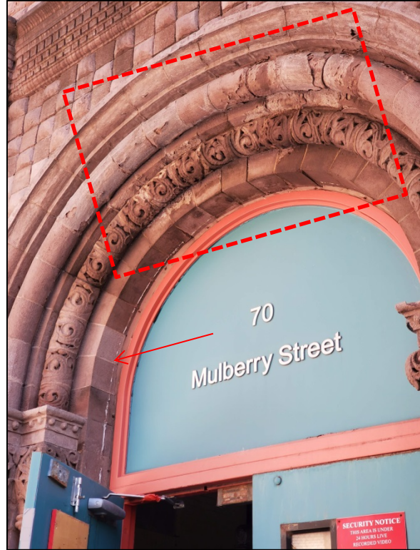
Figure 5: Spalling in decorative archivolt within dotted line and strip of caulking indicated with red arrow, Mulberry Street.
