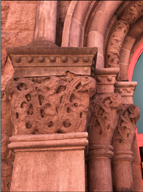
Figure 8: Engaged column, loss of detail, Mulberry Street entrance.
