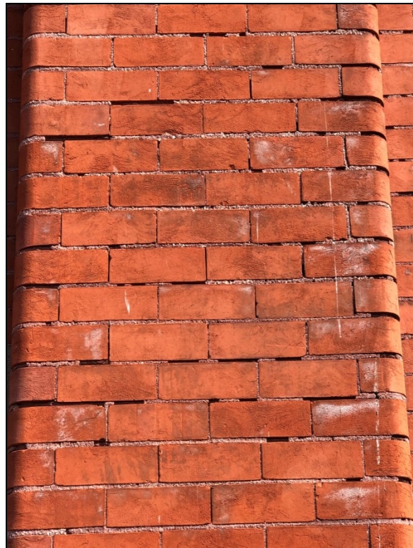
Figure 28: Open joints stair tower pilaster, Mulberry Street.
