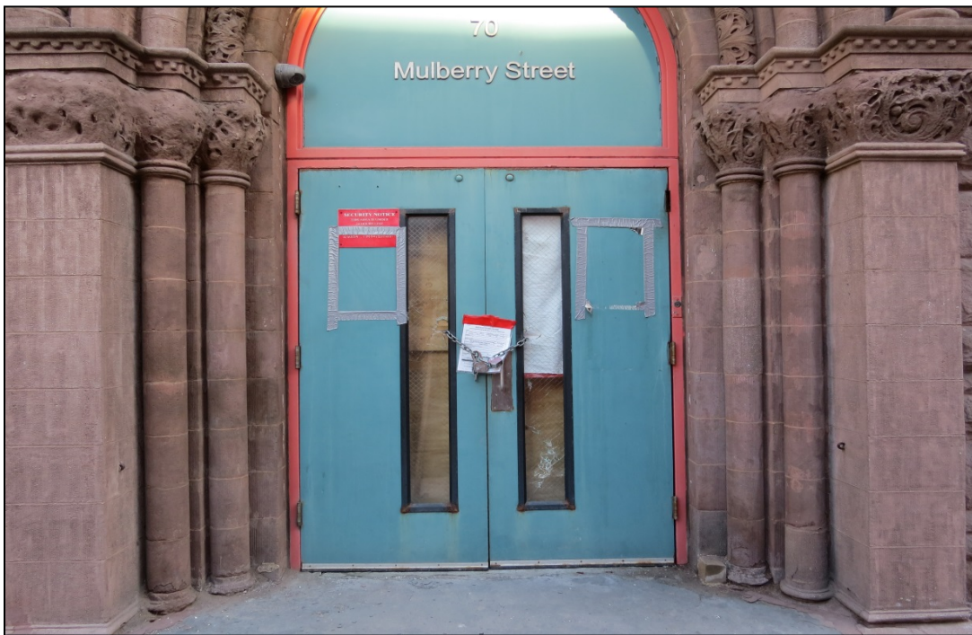
Figure 7: Bayard Street entrance loss of detail in capitals, spalling and delamination at base of engaged columns.
