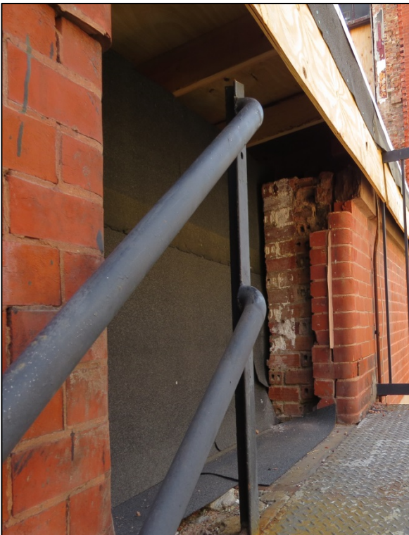
Figure 31: Masonry damage due to demolition, top of fire escape stairs, Mulberry Street.
