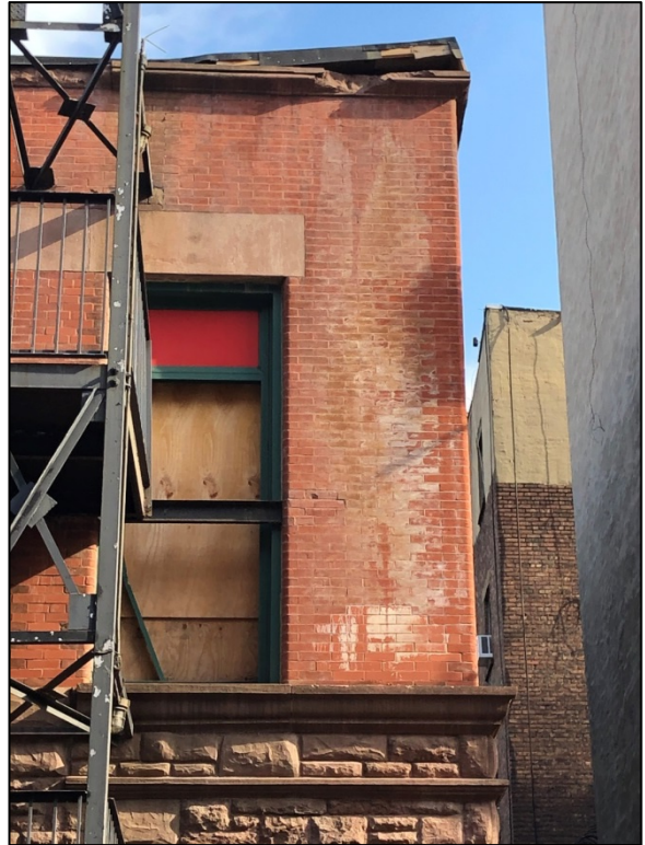
Figure 34: Damage and efflorescence, at the corner of Bayard Street.
