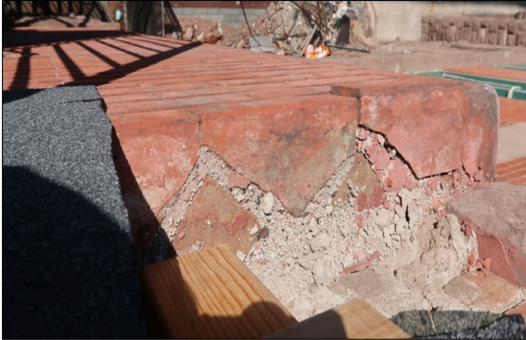
Figure 19: Looking down from above Pressed Brick in a stretcher bond with clipped brick bond to back-up masonry wall, Bayard Street.
