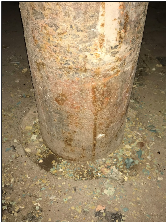
Figure 39: Missing cast iron column base.
