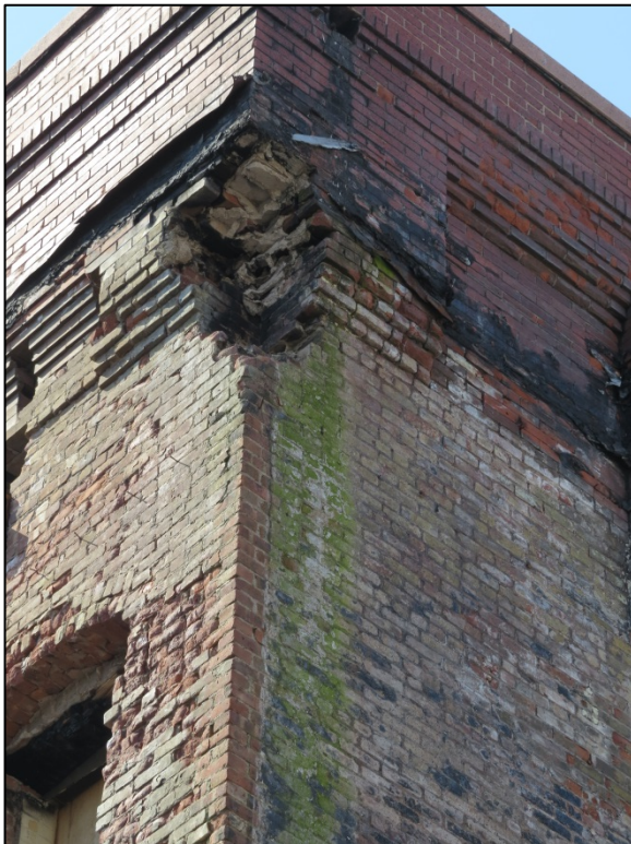
Figure 27: Northeast interior corner with brick loss damage and biological growth.
