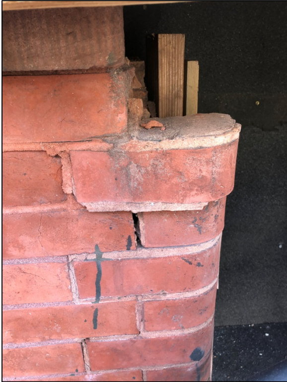
Figure 21: Displaced bullnose brick at fire escape, Mulberry Street.
