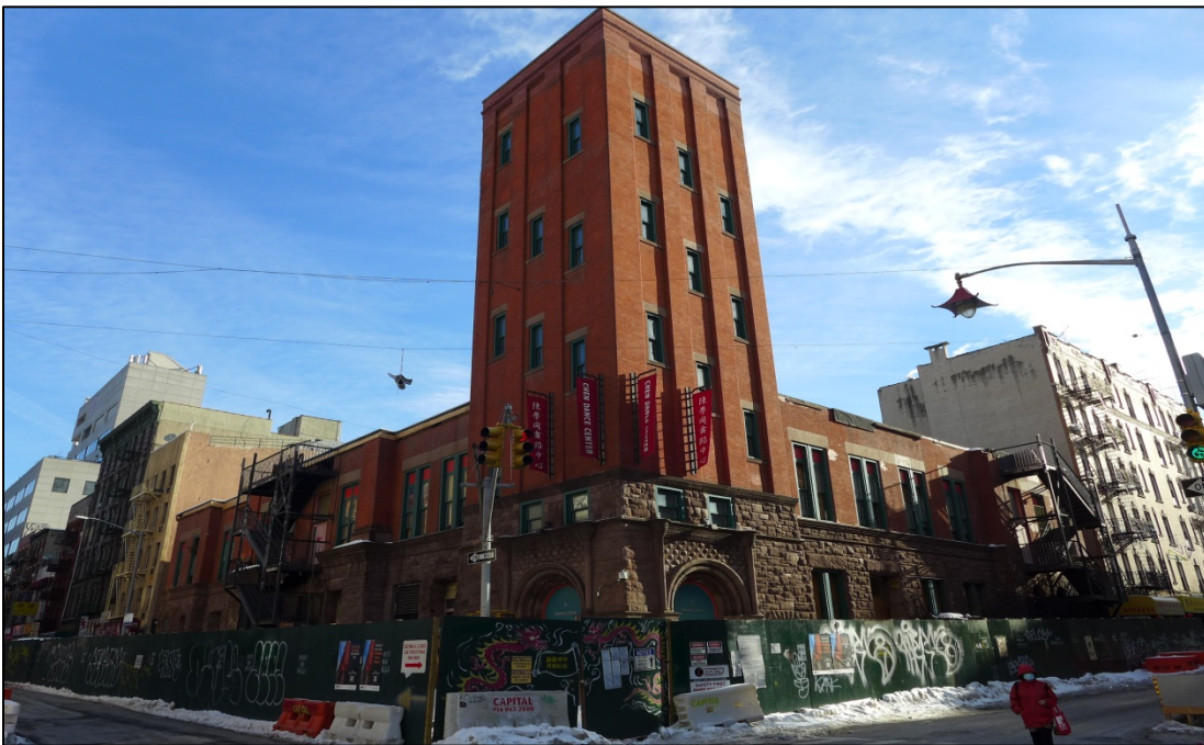
Figure 2: 70 Mulberry Street after fire and demolition.
