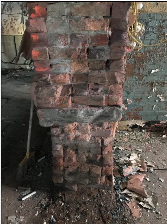
Figure 43: West elevation wall demolition damage.
