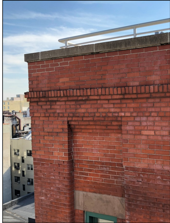
Figure 22: Replacement masonry at top of stair tower, Mulberry Street. Note the gray pointing mortar.
