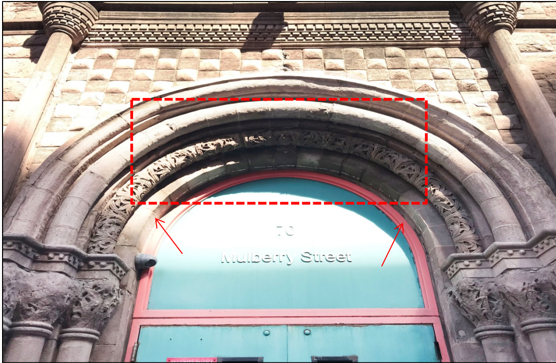
Figure 6: Spalling in decorative archivolt within dotted lines and strip of caulk indicated with red arrows, Bayard Street.
