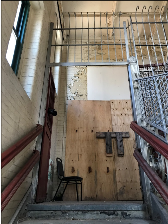
Figure 45: Fifth floor stair tower with peeling paint.
