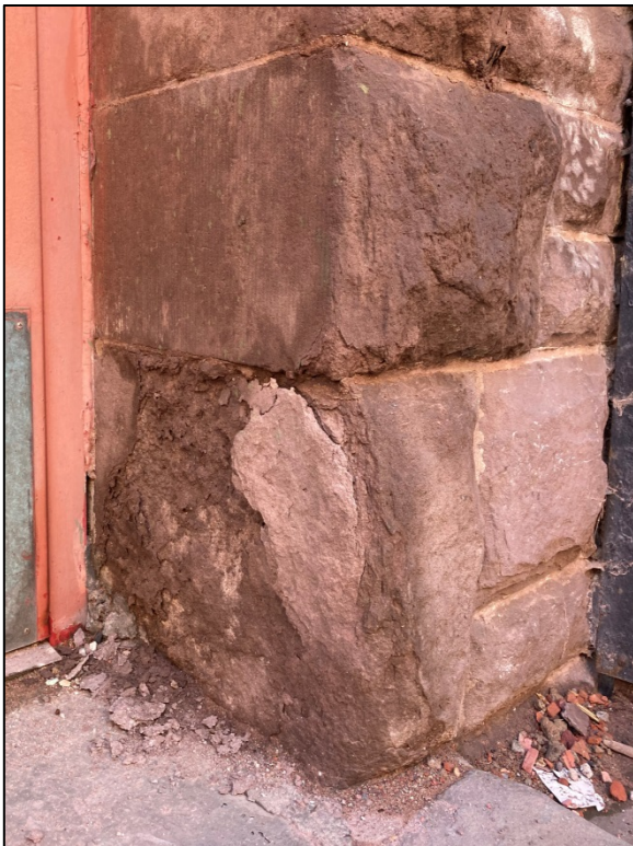
Figure 14: Delamination at base of side door entrance, Mulberry Street.
