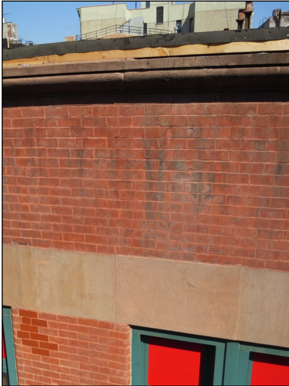
Figure 33: Atmospheric soiling and efflorescence, Bayard Street.
