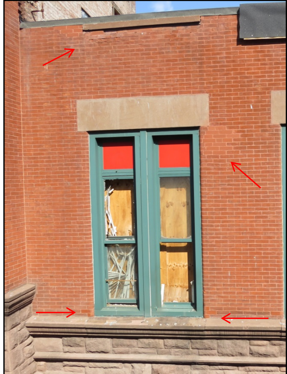
Figure 36: Infill, damaged, and missing masonry indicated with arrows, Bayard Street.
