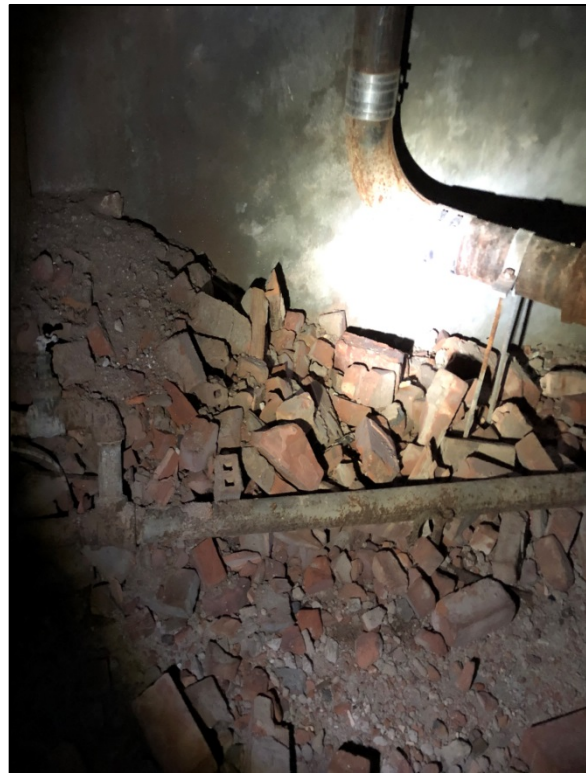
Figure 44: Pressed brick pile in basement.
