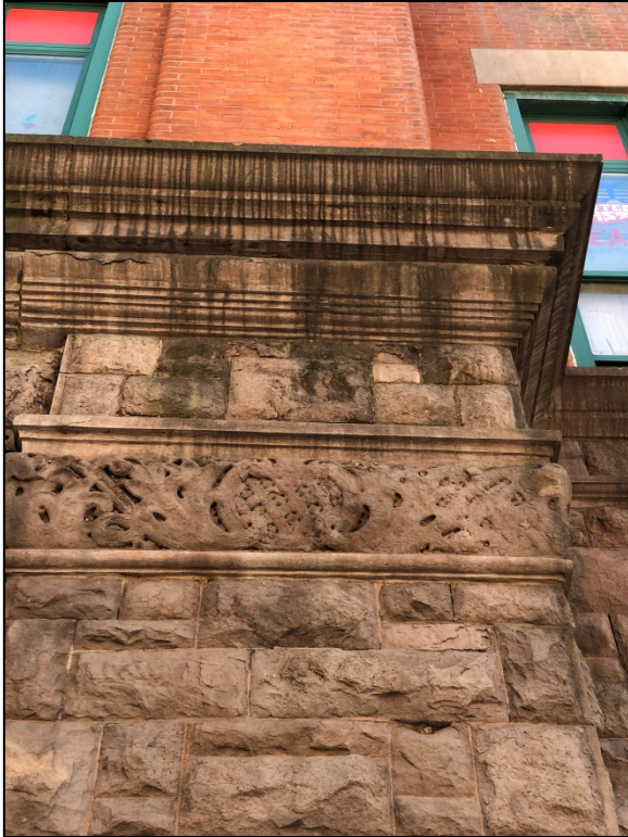
Figure 12: Biological growth and atmospheric soiling above side door, Mulberry Street.
