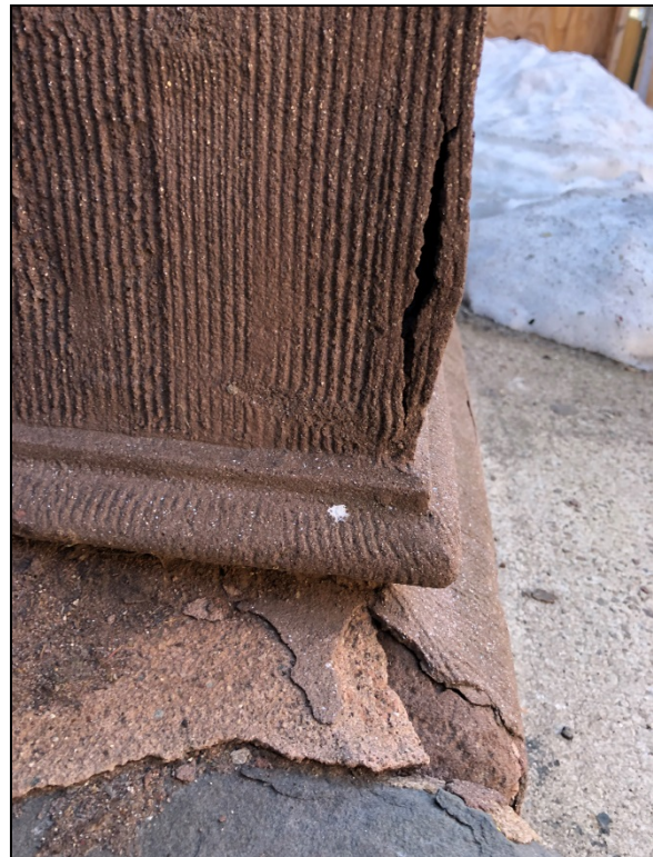
Figure 11: Spalling and delamination at bottom of column on the south side of Mulberry Street entrance.
