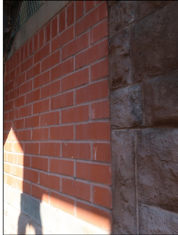
Figure 17: Non-matching infill brick repair behind fire escape, Bayard Street.
