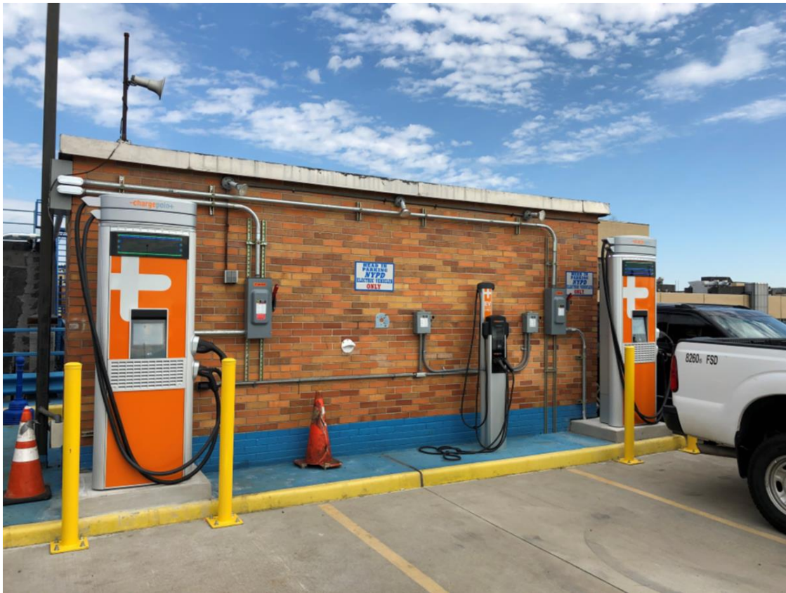
Electric vehicle chargers available for NYPD electric units.
