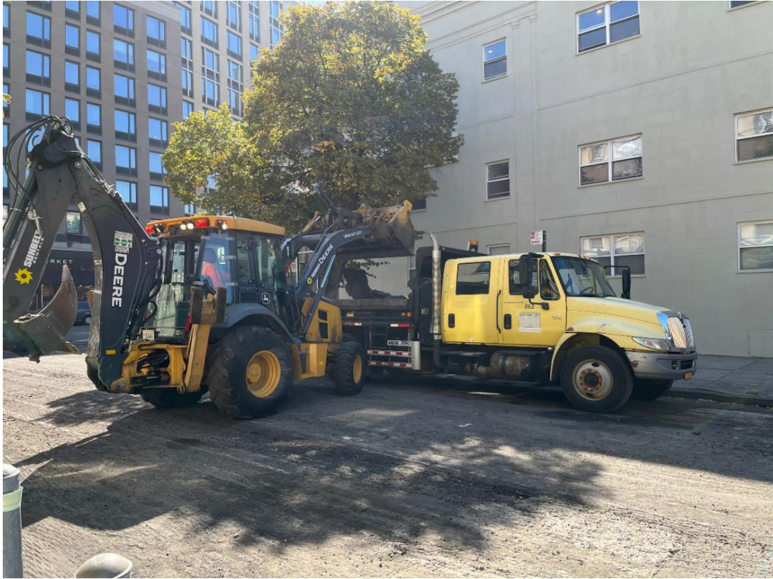
Front End Loader removing old asphalt and placing into DOT Dump Truck.
