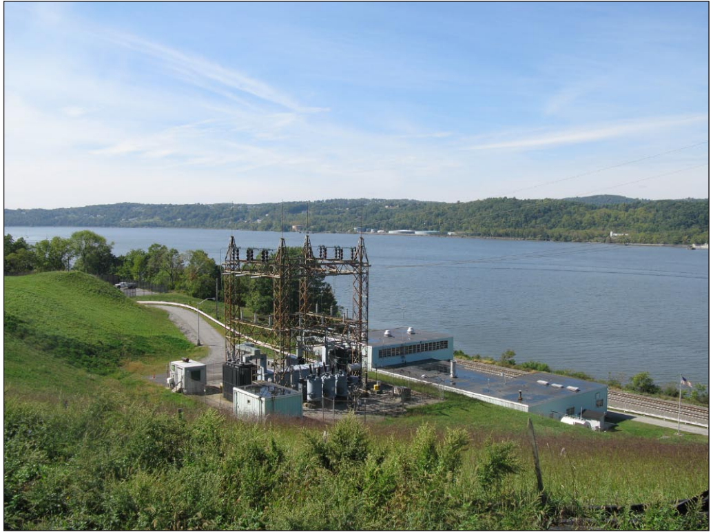
Substation and southwest building facing southwest 11
