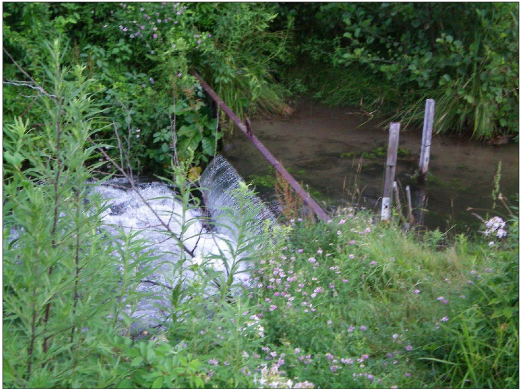
Weir in Segment 3 located upstream of the intersection of River Road and the Roseton/Danskammer transmission line access road 6
