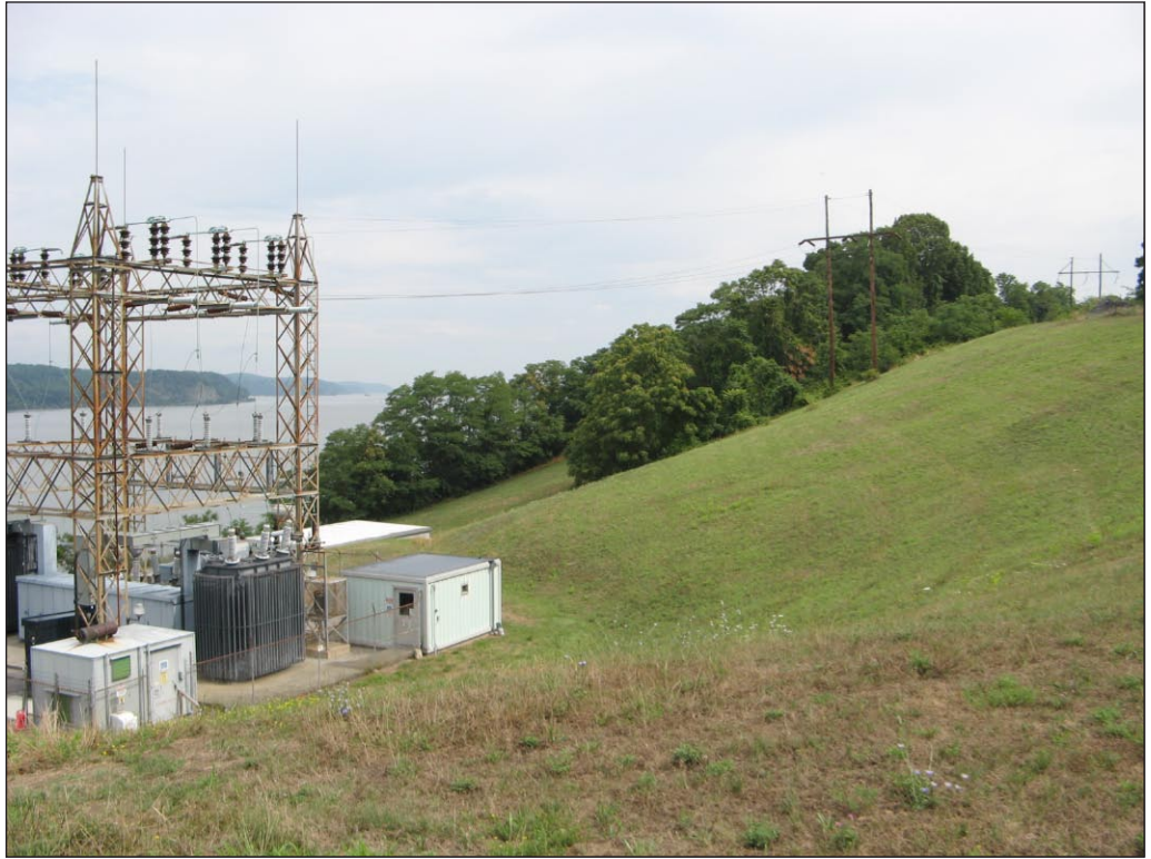
Northwest tree stand and substation facing north-northwest 7
