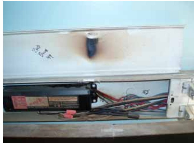
An old ballast that exploded unexpectedly.
