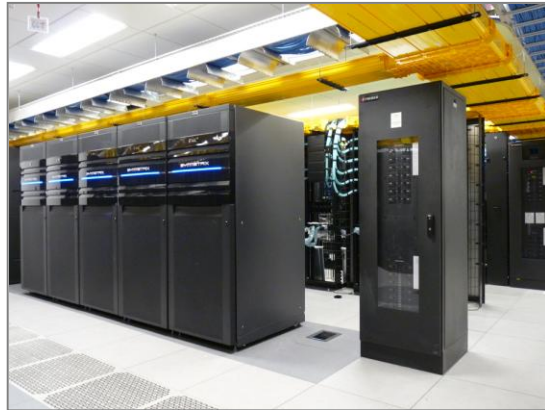
CITIServ: State-of-the-art citywide data center facility in downtown Brooklyn’s 2 MetroTech Center.
