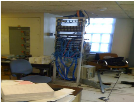
BEFORE CITIServ: Suboptimal agency data center facility at 345 Adams Street
