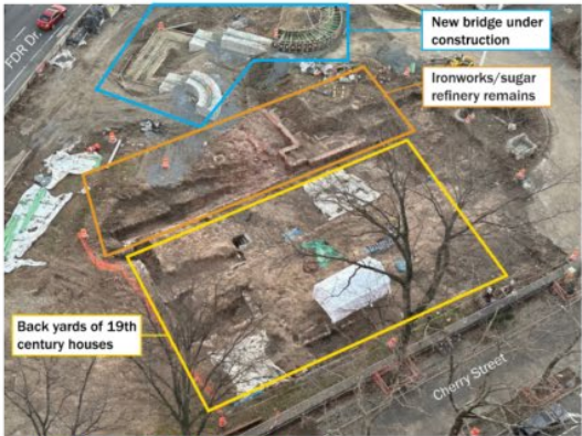
Aerial view of Corlears Hook Park construction site Photo credit: Friends of Corlears Hook Park
