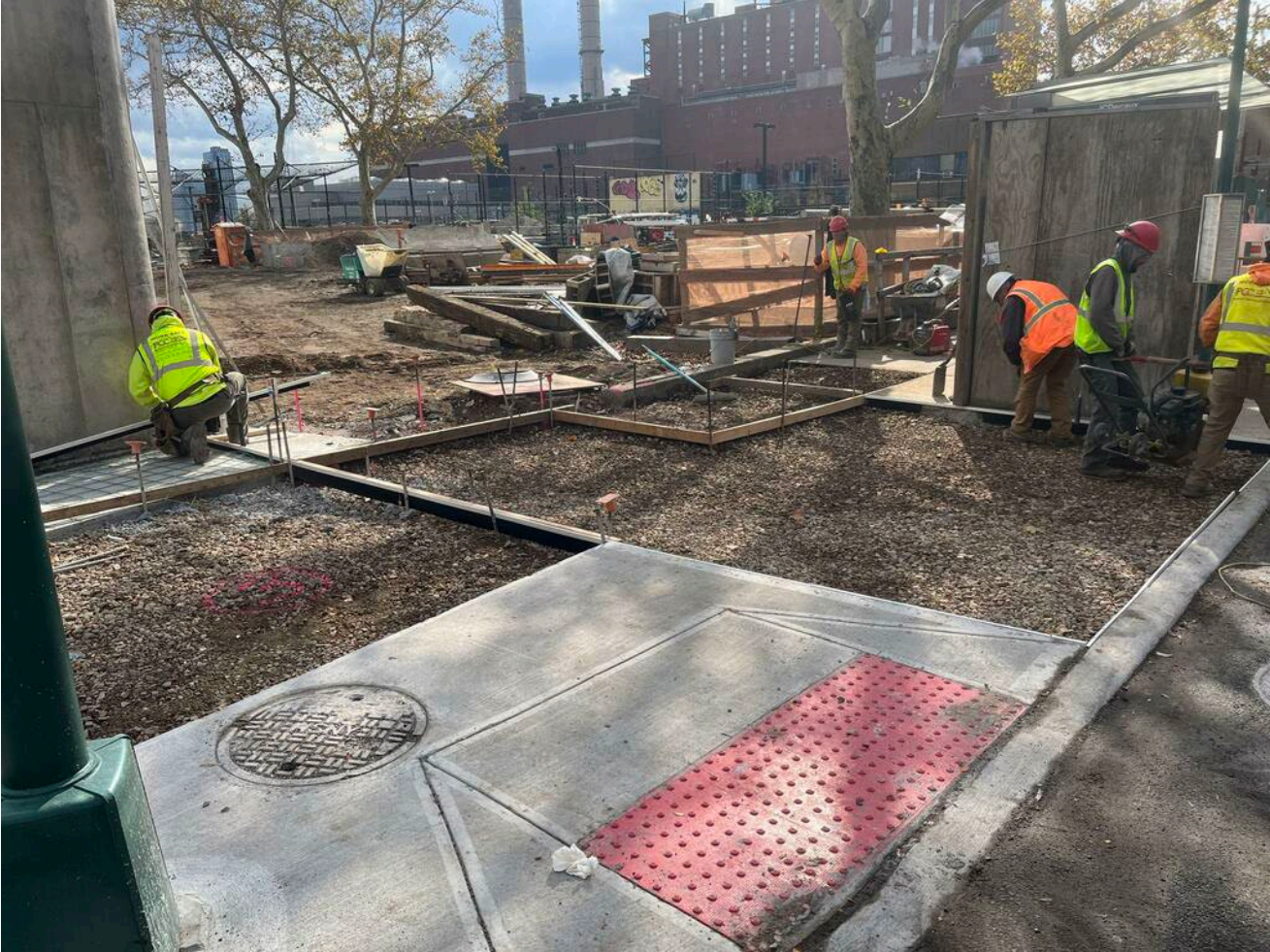
Preparation for Sidewalk Restoration at 18th Street (Murphy Brothers Playground Entrance) – November 2023
