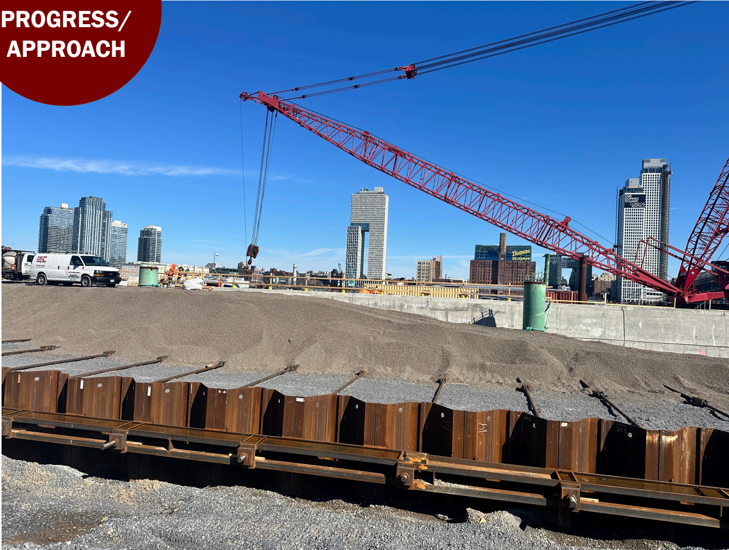
Buried flood wall, tiebacks, and cutoff wall north of Williamsburg Bridge – March 2024
