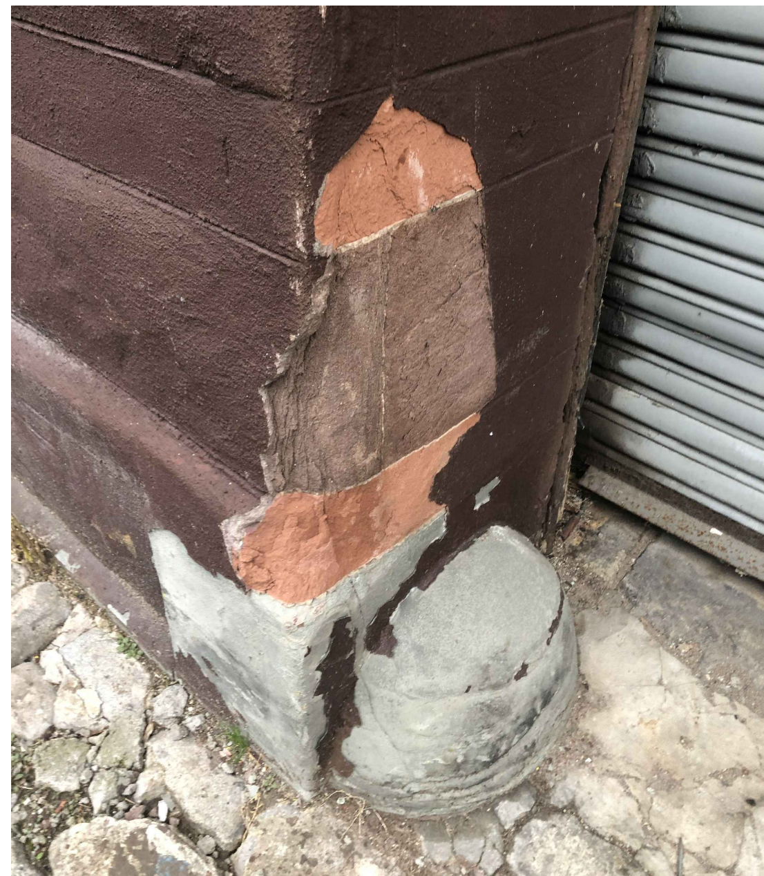
EXISTING RUSTICATED BASE
