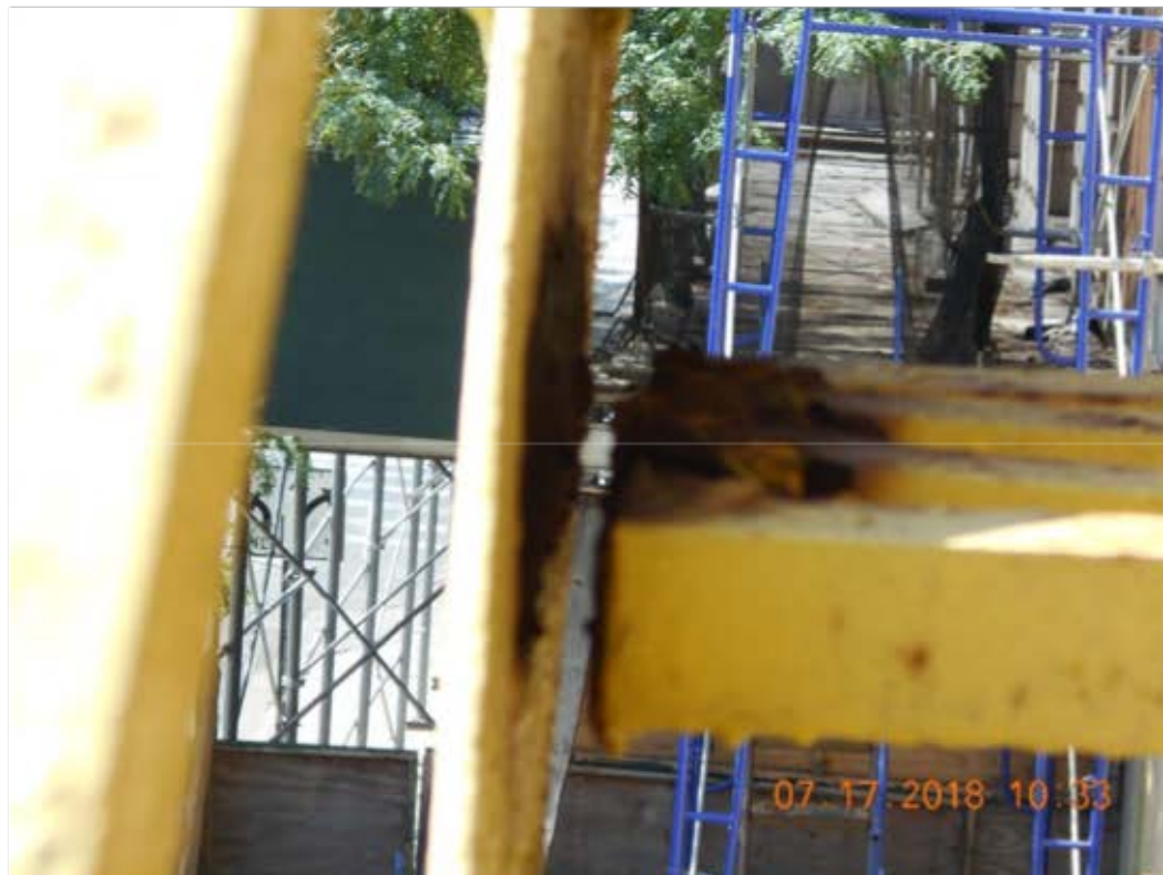
Figure 6 – Note complete separation and lack of load path between stair tread and stringer.
