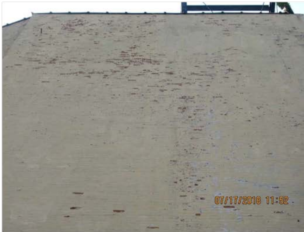
Figure 6 – Close-up of spalling conditions of North theater exterior wall.
