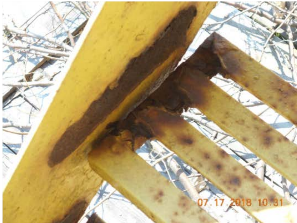
Figure 5 – Stair stringer and stair tread. Failure of tread connection to the stringer.
