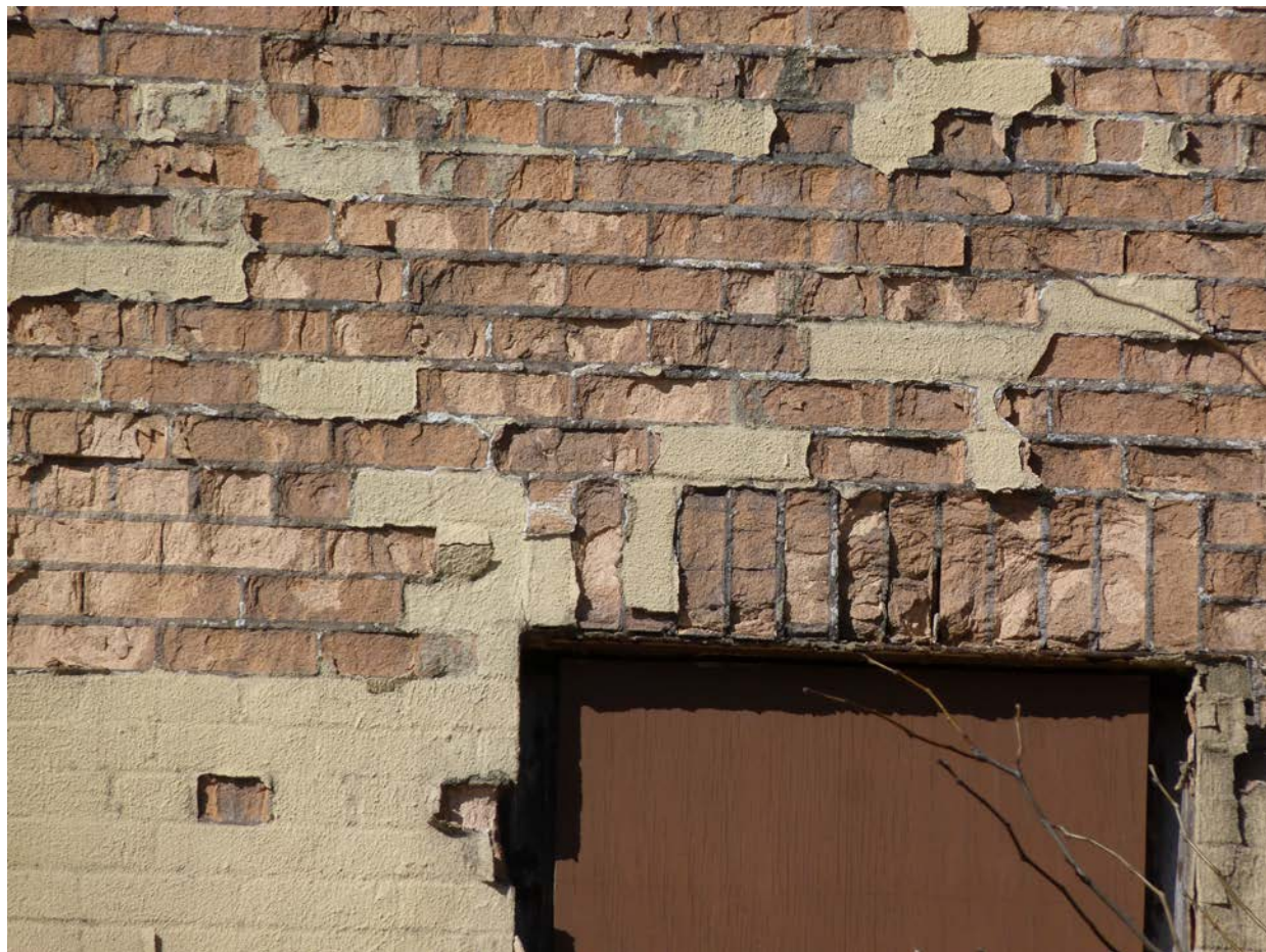
Spalled brick faces
