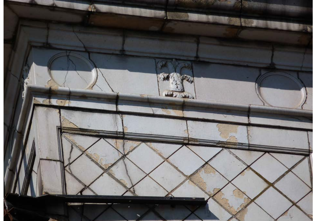
Cracked terra cotta
