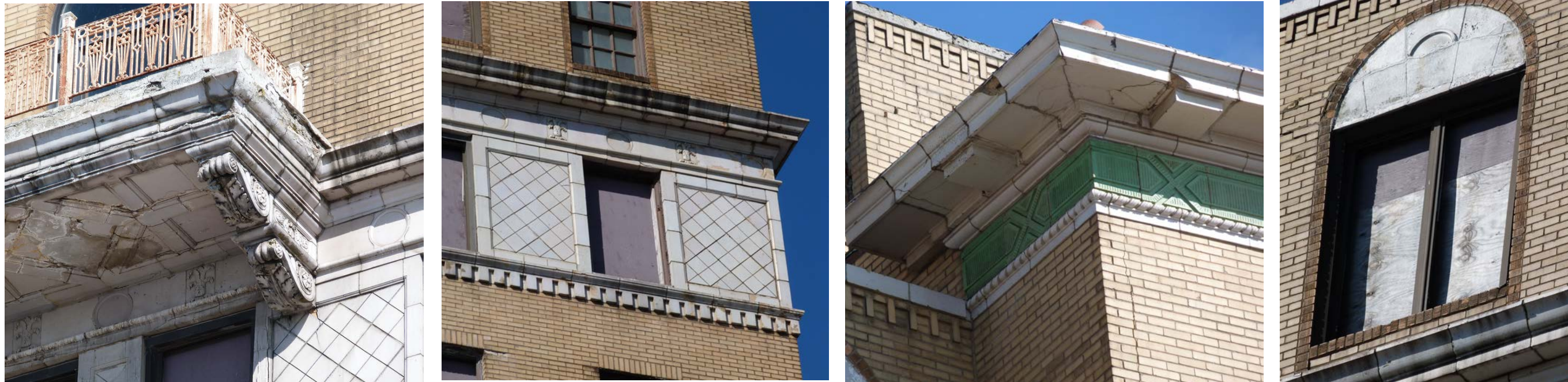
EXISTING CONDITIONS OF TERRA COTTA
