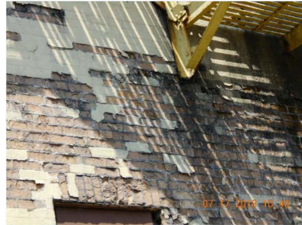
Figure 7 – Deterioration and spalling of masonry wall in area of stair support bracket.
