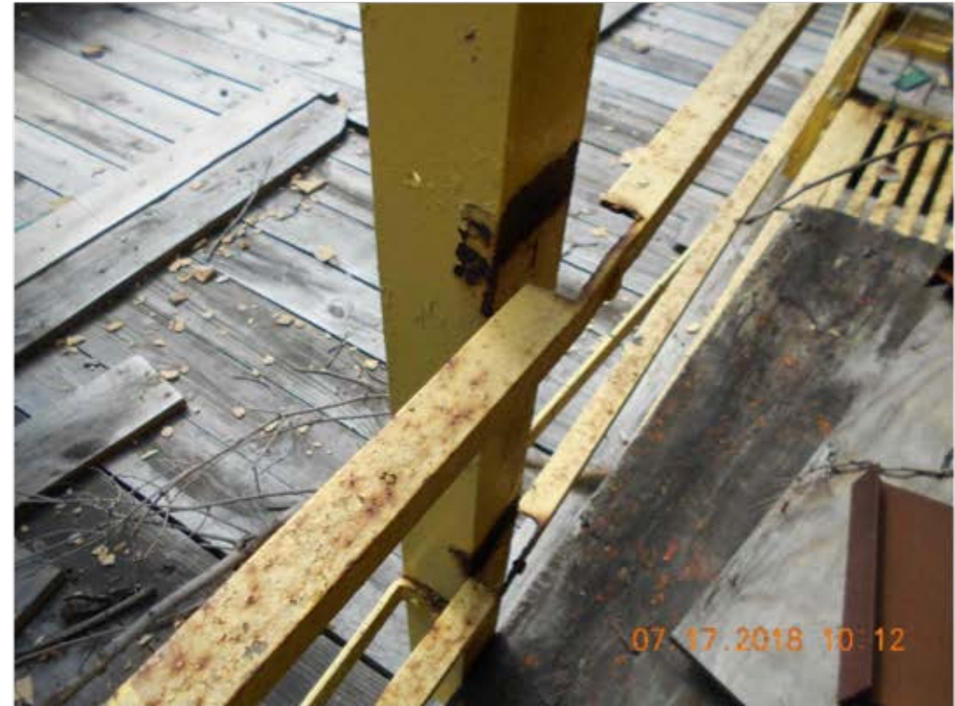
Figure 3 – Main landing. Failure of railing connection to support.
