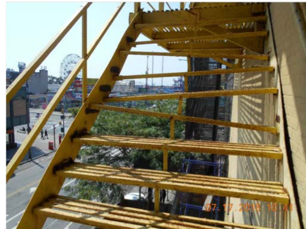
Figure 8 – Inherently unstable treads and unbraced stringer
