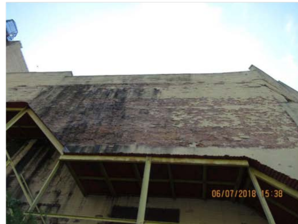
Figure 8 – Close-up of spalling conditions of East theater exterior wall.
