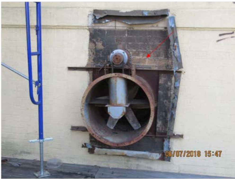
Figure 9 – Spot location on East theater wall showing un-coated wire faced brick.
