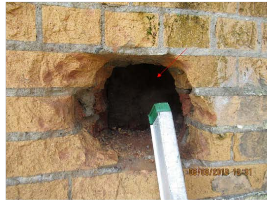
Figure 11 – Additional East wall probe within heavily spalled masonry with steel column beyond which was also observed to be wet.
