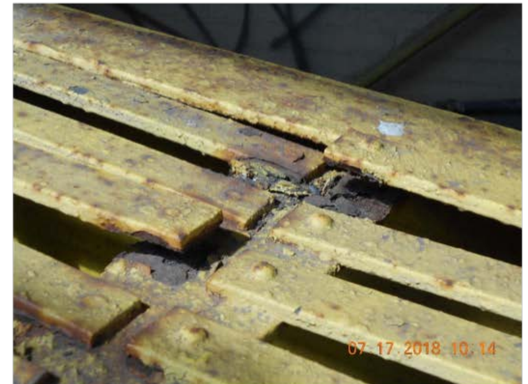
Figure 4 – Main landing. Failure of bar connection to support.
