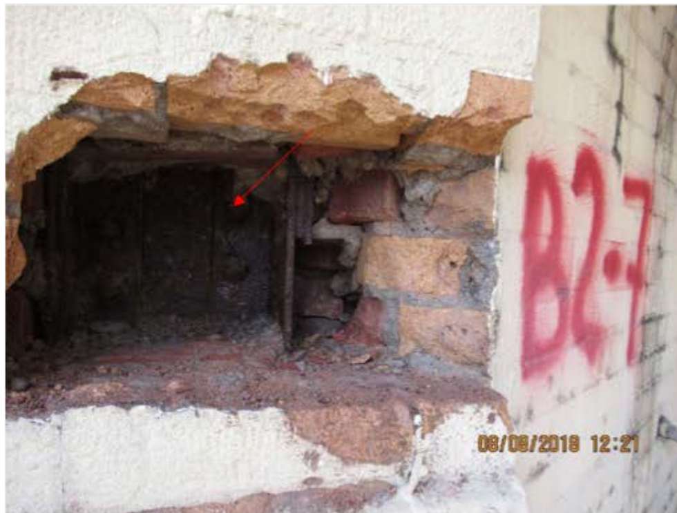
Figure 10 – East wall corner probe with steel column beyond which was observed to be wet.
