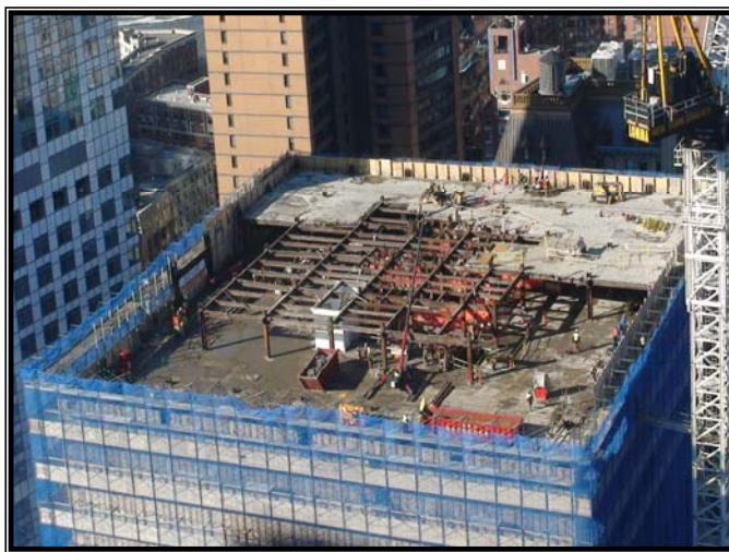
Figure 8. Deconstruction at 130 Liberty Street, provided by the LMDC at a regular report to the WTC Redevelopment Committee in January 2010.
