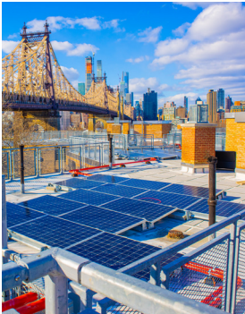
Commercial Solar installed at Queensbridge Houses
