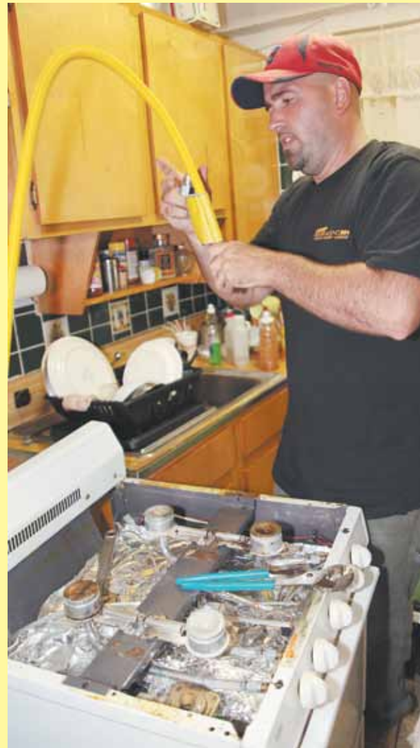
NYCHA plumber Mike Reed checks a gas stove as part of NYCHA’s response to a large gas outage in upper Manhattan in August 2011.
