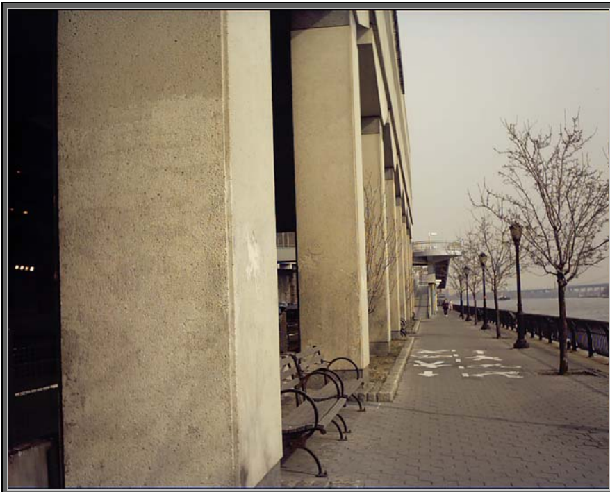
2. View looking north along the esplanade showing footing columns for the East Wing.
