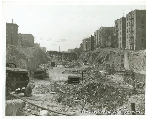
The Building of the Cross Bronx Expressway Source: Lehman College Library (CUNY)
