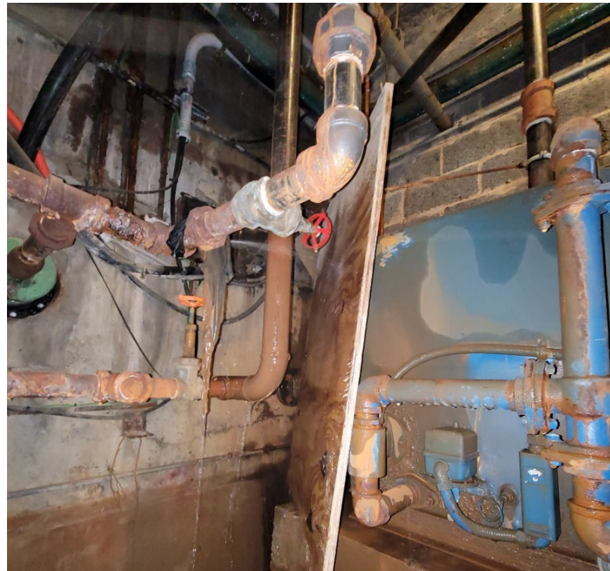
Water leak requiring repair
