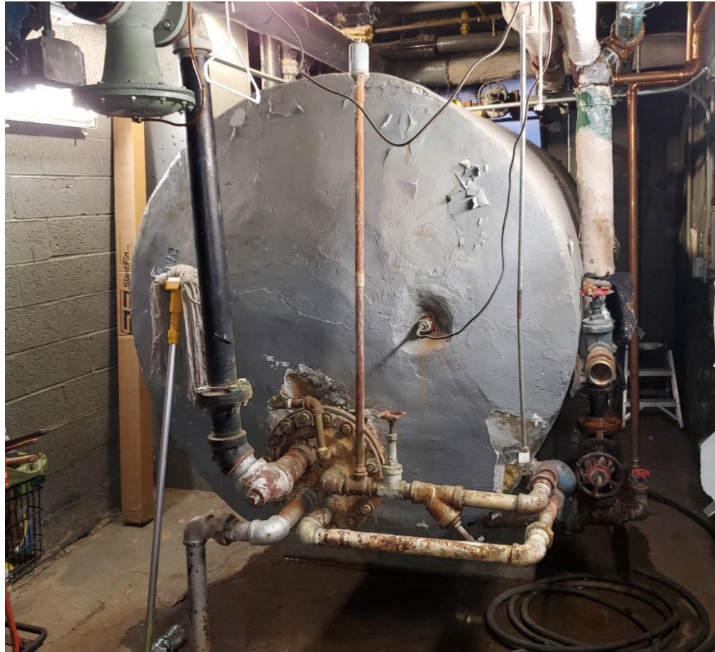
Insulated hot water tank
