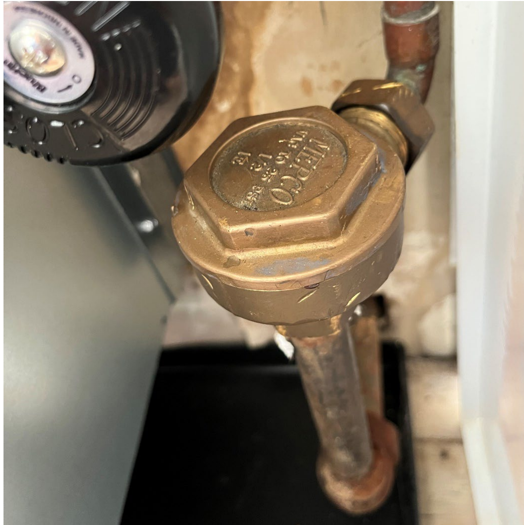
Thermostatic steam trap in a dwelling unit
