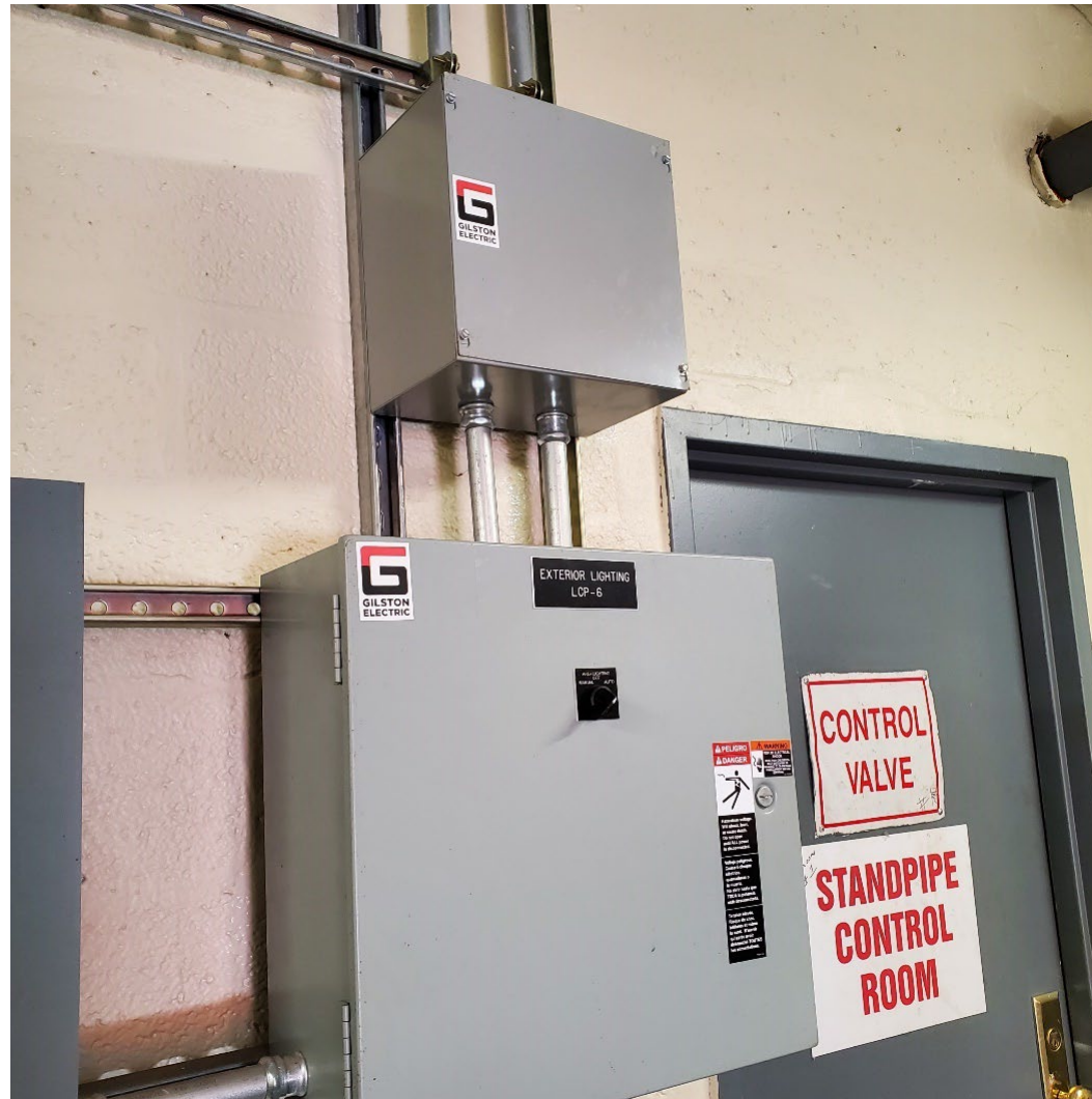
Exterior Lighting Controls
