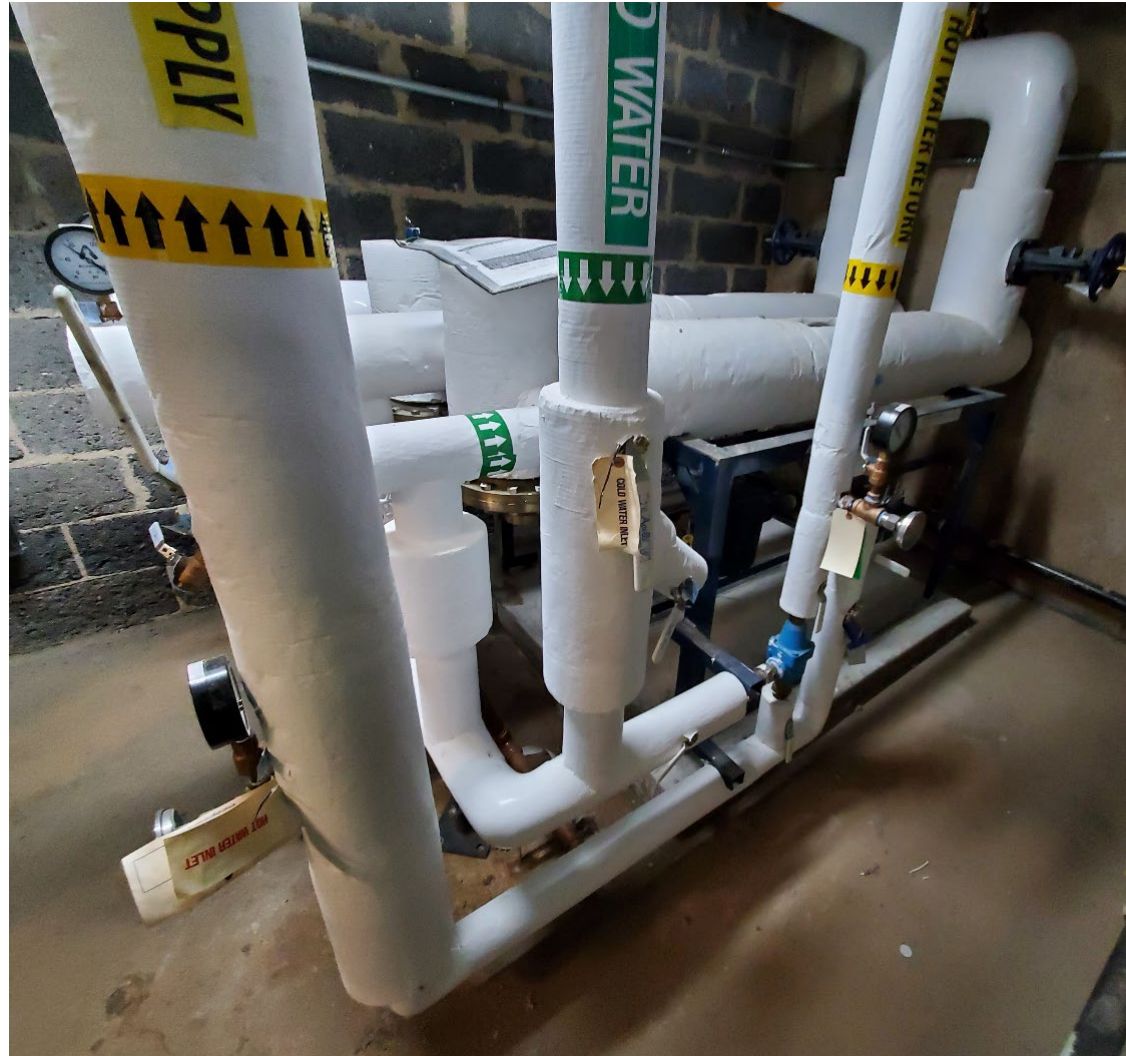
Insulated and labeled water pipes
