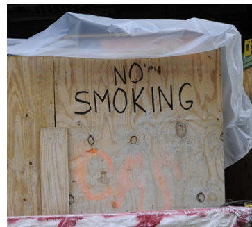
Unacceptable Warning Sign
