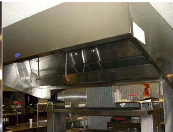
TYPE I HOOD WASH HAS PLENUM DOORS
